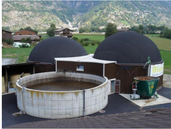
Biogasanlage in Visp
